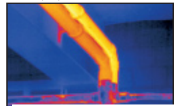
Overheat in process monitoring
